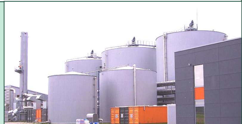
Anaerobic digesters at the Lübeck Waste Treatment Facility a mechanical biological treatment plant.
